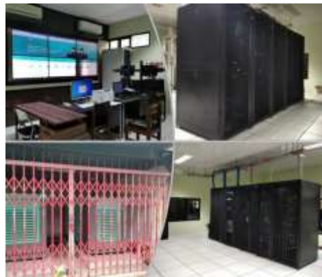
Figure 4. Data Centre Space
