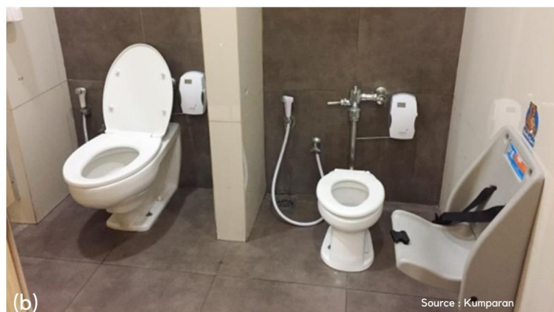
Figure 2 Illustration of sanitation facility for children (a) Sink, (b) Family Toilet
