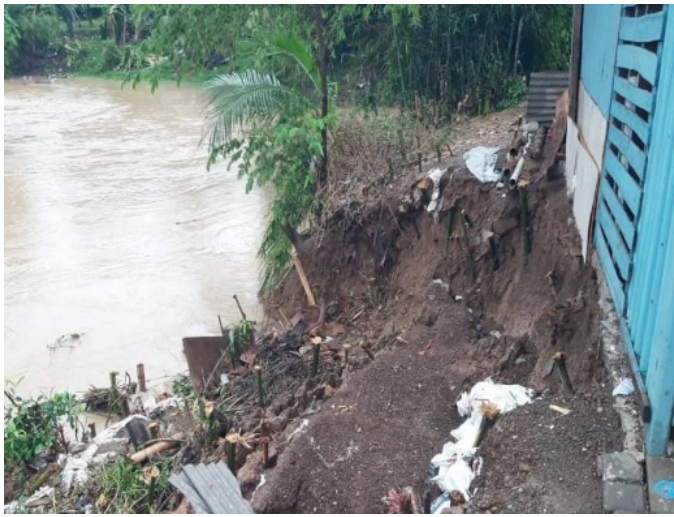
Picture 4. The documentation of the landslide in Wadas Village. 41
